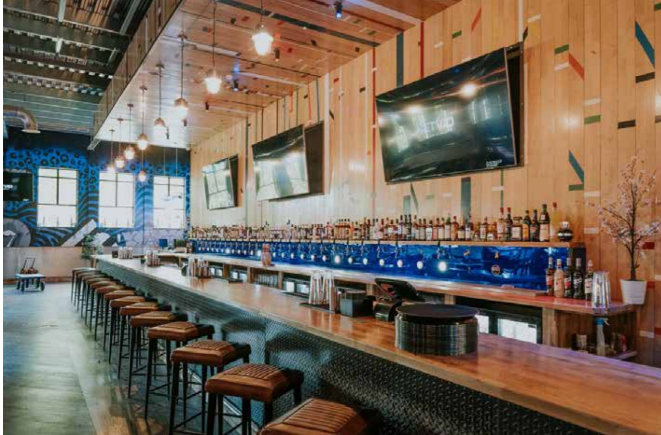
Three large displays over the bar area and nine further screens are driven and controlled by Netvio JP4 AVoIP
